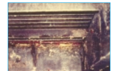
After system cleaning – the consequences of microbial contamination (corrosion as a result of microorganisms) can clearly be seen
